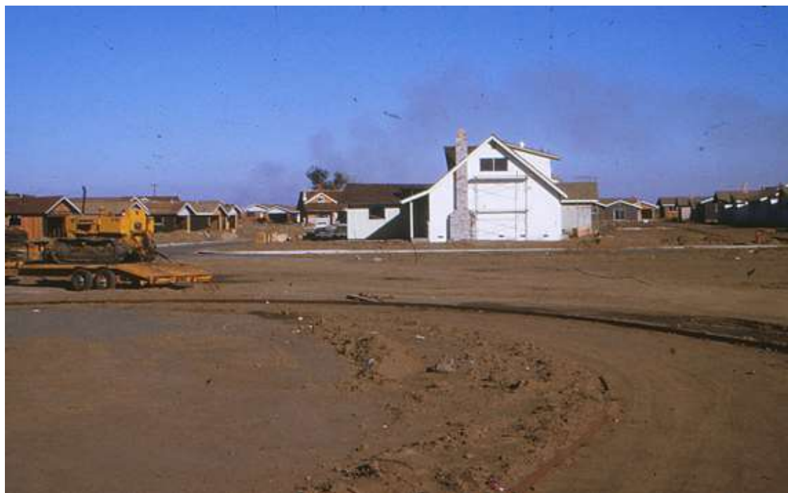
Figure 17: Grinnell Drive in Davis Manor No. 17 under construction in 1972 (courtesy of John Lofland).
